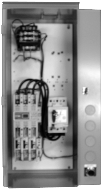
Irrigation Pump Panel
