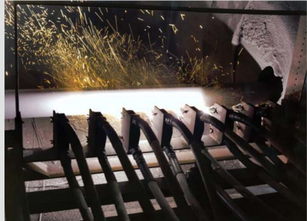
Sermatech has developed an automated process for applying the TSA Coating Protection System to piping up to 75 feet long.
