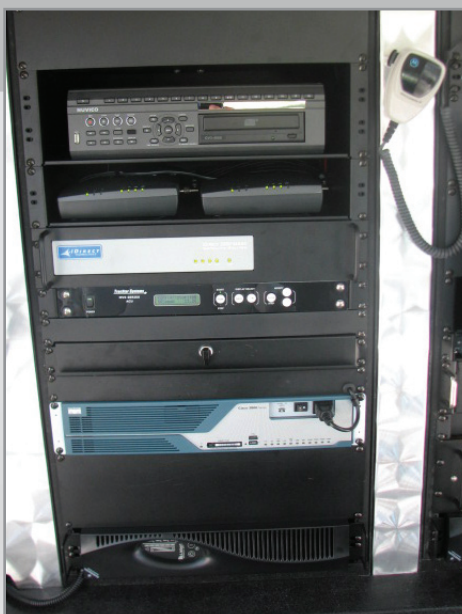
19" electronic rack with DVR, Satellite modem and Cisco router.
