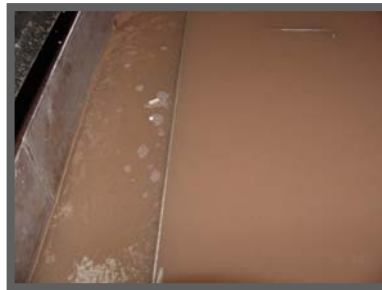
Influent to HIFLOAT DAF System
