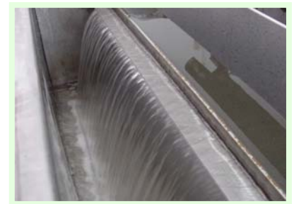
Effluent from HIFLOAT DAF System
