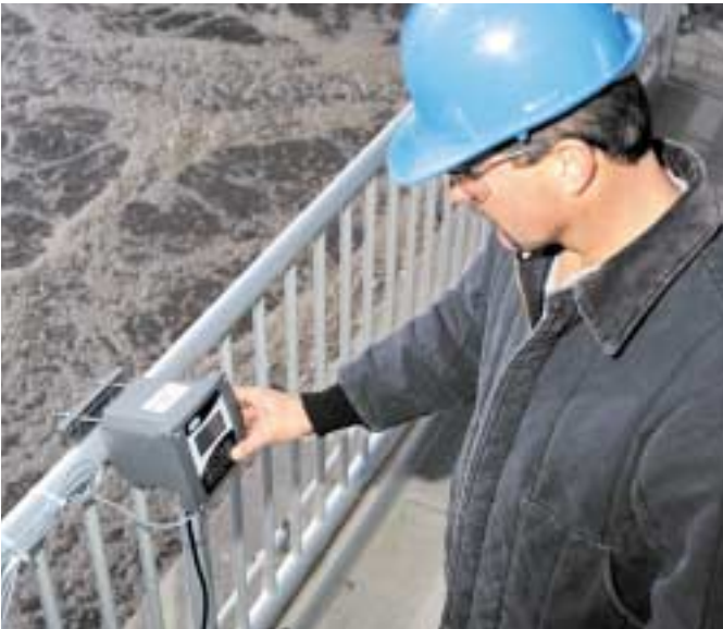
The sc100 controller has a big and bright display and clearly arranged pushbuttons for simple operation.
