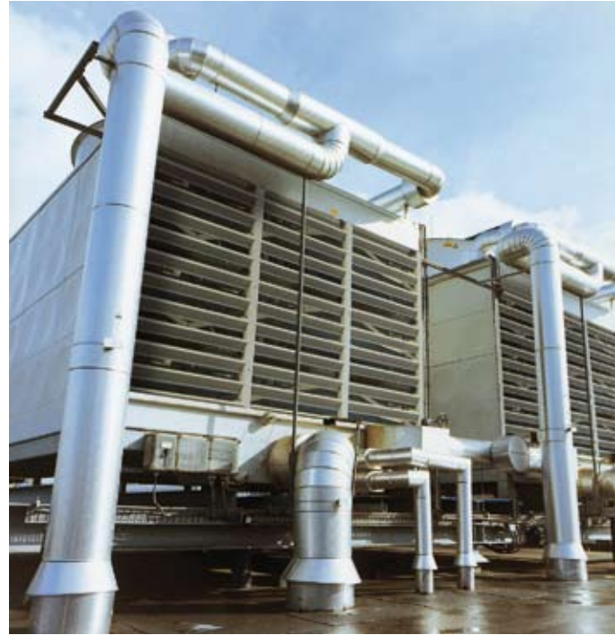
Cooling Tower type XL 2.320 Chemical Plant in the Netherlands
