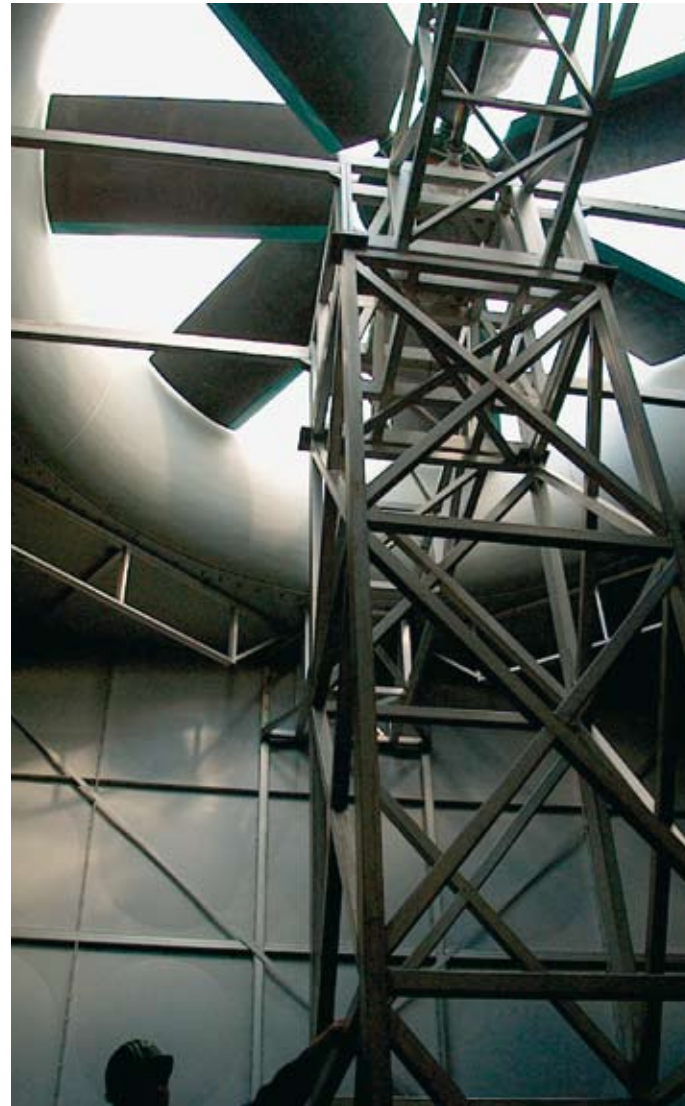
Skeletal and fan of the Cooling Tower from the inside view
