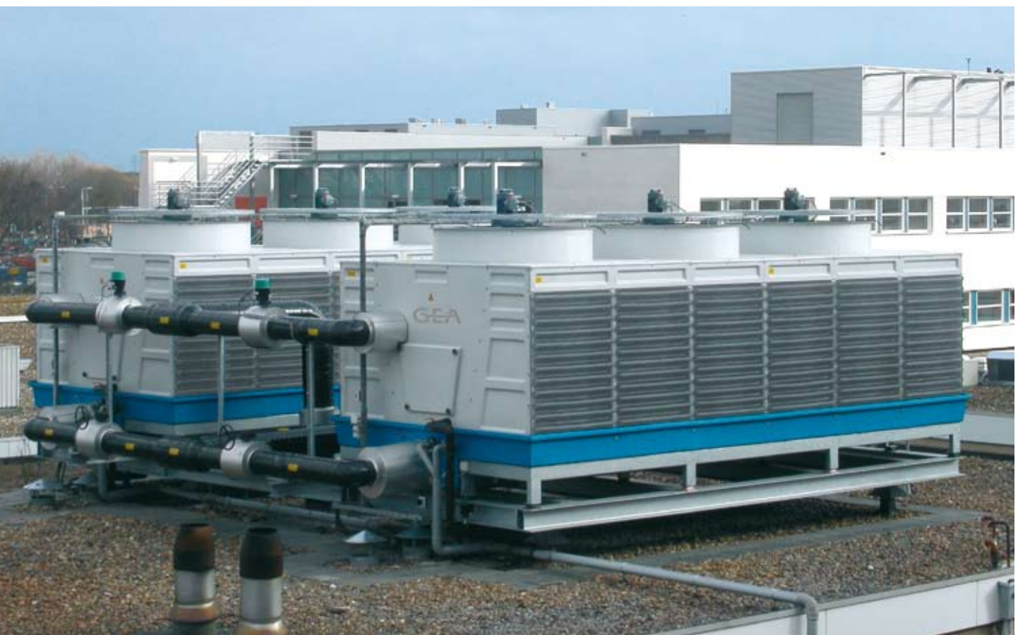
Cooling Tower type XT 2.720 Hospital in the Netherlands
