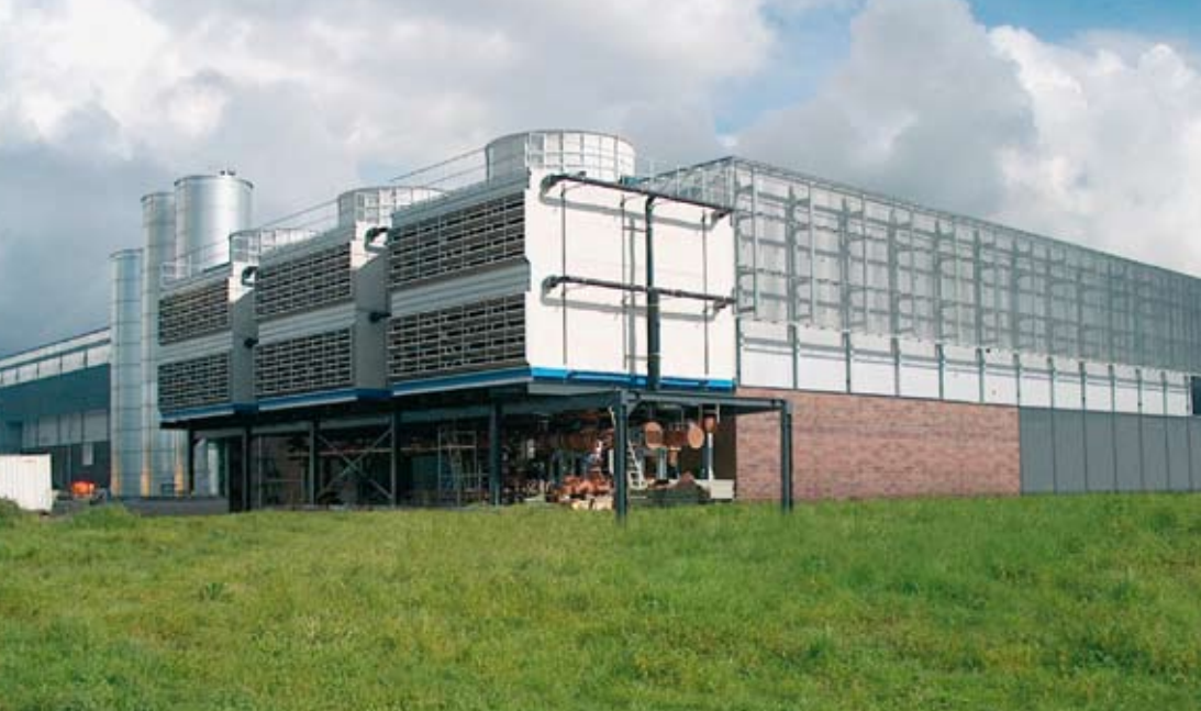
Cooling Tower type 3 XMS 2.720 Telephone-/Communication center in the Netherlands
