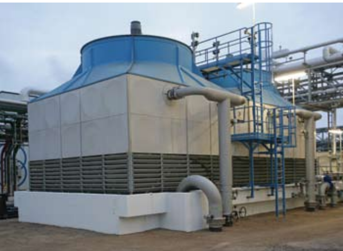
CMDR cooling tower type 380 Chemical Plant in Germany
