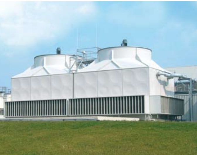
CMDR cooling tower type 460 Car manufacturer in Germany
