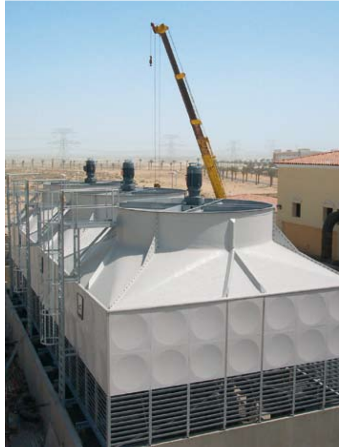
CMDR cooling tower type 630 Green Community in United Arab Emirates
