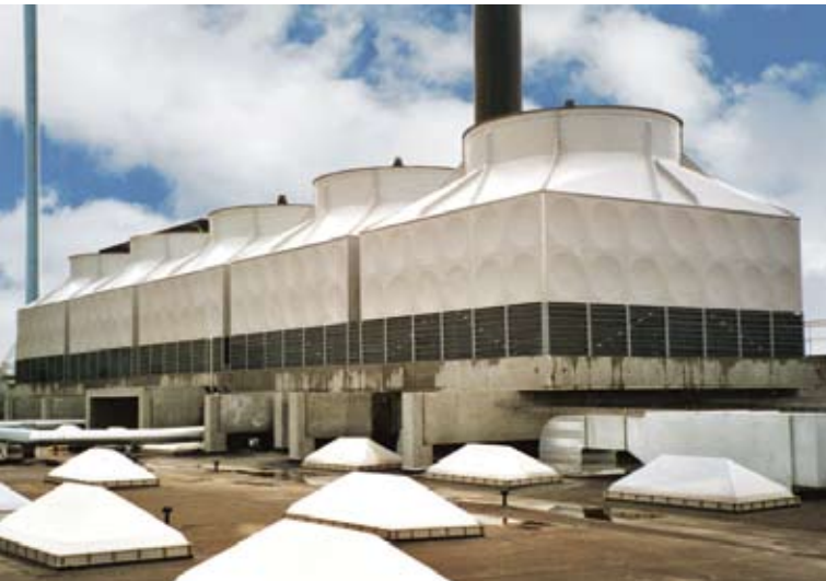
CMDR cooling tower type 630 Lysine factory in Denmark
