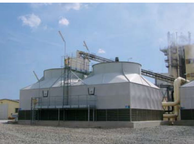
CMDR cooling tower type 630 Chemical Plant in Germany
