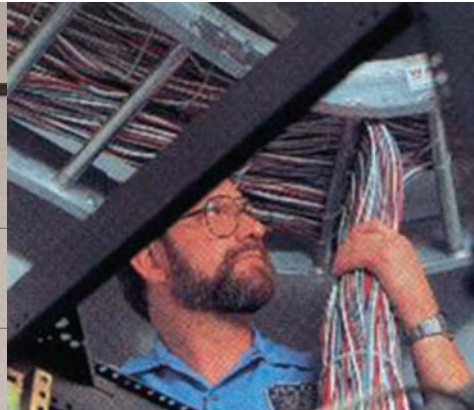
Overhead cable distribution is difficult to service, manage and reconfigure.
