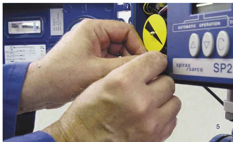
Commissioning a positioner component of the QuickHeat
