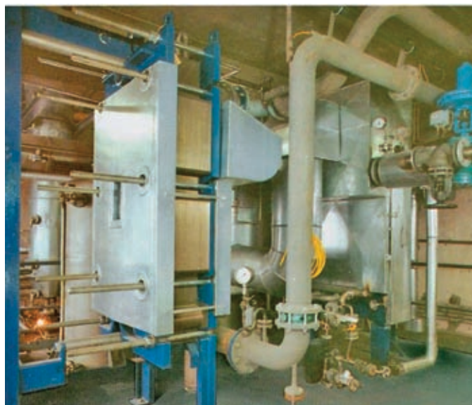
Vegetable Oil Evaporator with the Simultaneous Recovery of Extraction Solvent
