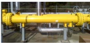
Shell and Tube Heat Exchanger: Before
