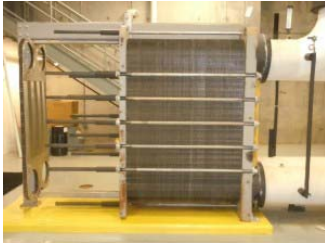
Plate and Frame Heat Exchanger: Before
