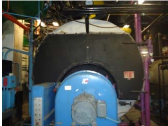
Scotch marine boiler – before
