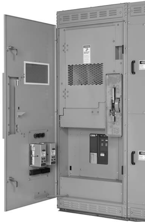
Indoor Medium Voltage Switch and Fixed Breaker — MSB
