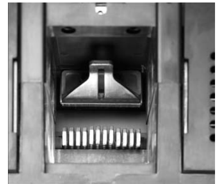
Magnum DS Breaker Contacts (Arc Chutes Removed)
