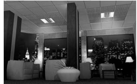
Radiator diffusers surround light fixtures in a hotel lobby ceiling.
