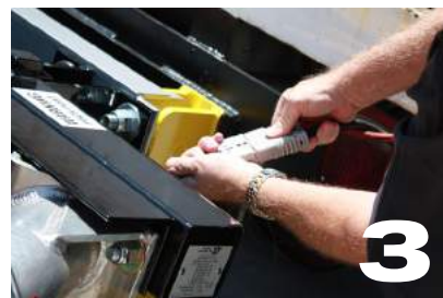
Plug in electrical connections
