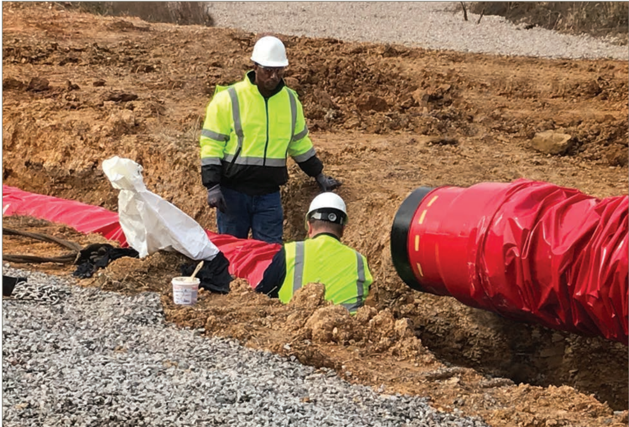
Joint assembly can be readily performed by two workers in a trench and one worker on the backhoe.
