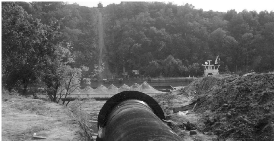
Bank installation in progress, where most of the work is performed on firm ground and the pipe is pulled across waterway by cable. (Note rail weights strapped on to create slight negative buoyancy of this size line pulled beneath barge traffic).
