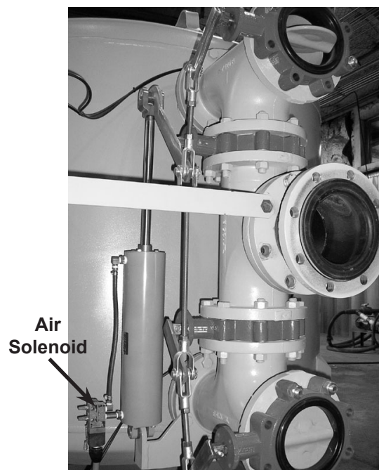
And in backwash position.
